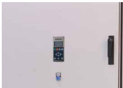
Lockable door prevents unauthorised access.
