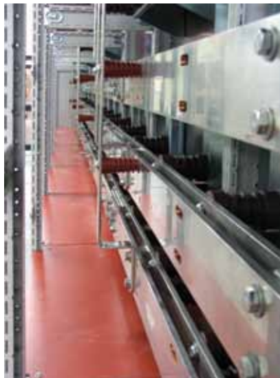
Horizontal bus bars can be engineered throughout the length of your panel. Insulated panels to isolate input and output bars are optional.
