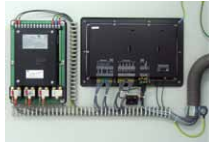
Fibre-optic cables isolate medium voltage and low voltage sections of the MVS and ensure 100% safety for operating personnel.
