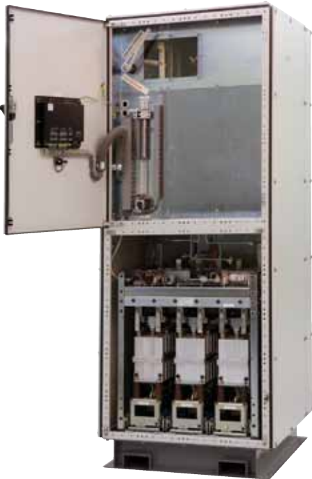
Front view of MVS panel with door open, MVS power assembly is located in lower section.
