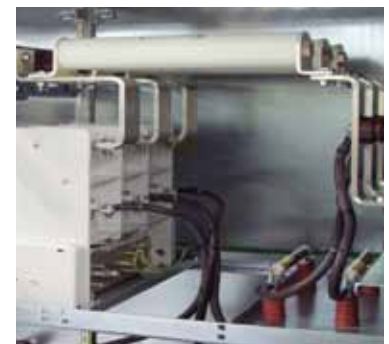
Contactor and fuse detail.
